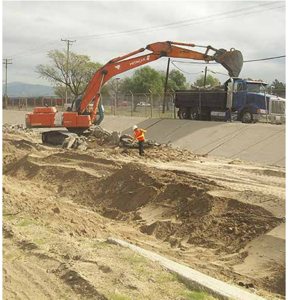
In 2018, crew demolished and removes damaged portions of the City Creek wash on the south side of Third Street to install new concrete panels through an IVDA rehabilitation project. City Creek is one of the primary drainage systems in the AGSP. Source: Highland Community News.
